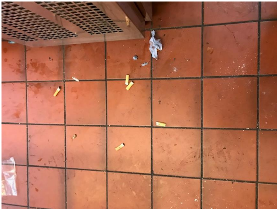
Ground Floor Kitchen - Cigarette butts on kitchen floor Photo taken Thursday 13th June 2019 at 12:23hrs
