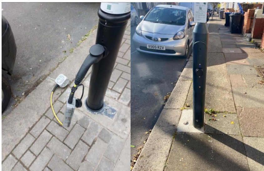
Examples of the EVCPs Installed within Bollards and Lampposts around the Borough (Source: LBB)
