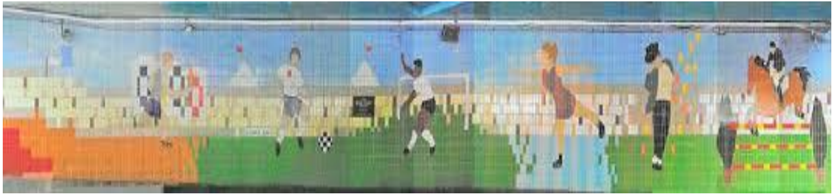
Tiles in underpass on eastern wall prior to installation of light boxes on either side of the plaque mural
