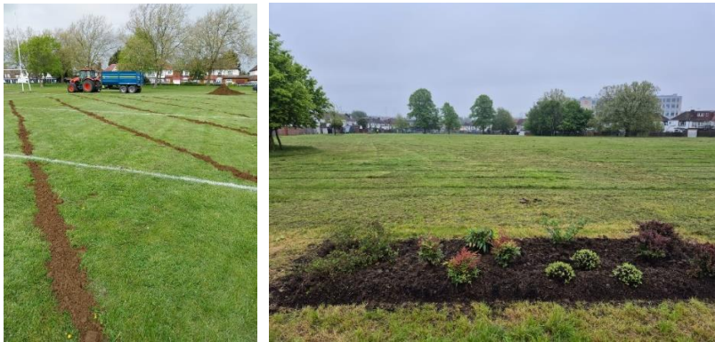
Figure 10 Images of Drain Lines repairs on Gaelic Football and Shrub bed installation in Heather Park
